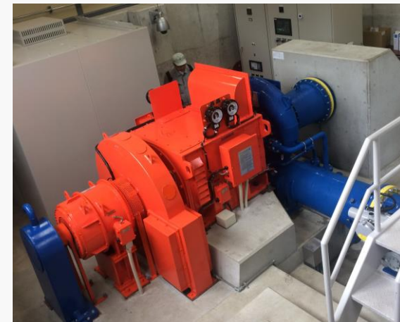
Micro hydro power generation facility
