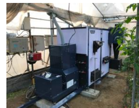
Biomass boiler installed at banana plantation
