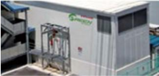
Onsite power generation facility at the Kobe Works
