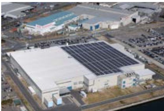
Nagoya Works: 750-kW power generation facility
