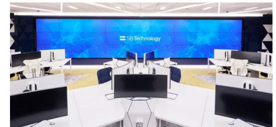
Security Monitoring Centre
