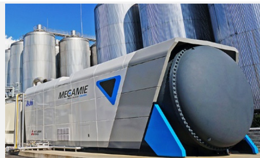
A fuel cell power generation system using biomethane gas generated from brewery wastewater
