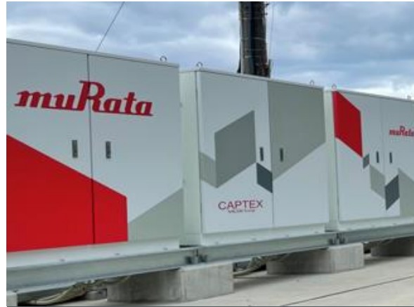
Power storage system that uses Murata cells
