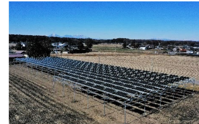
Moka City Solar Sharing Power Plant
