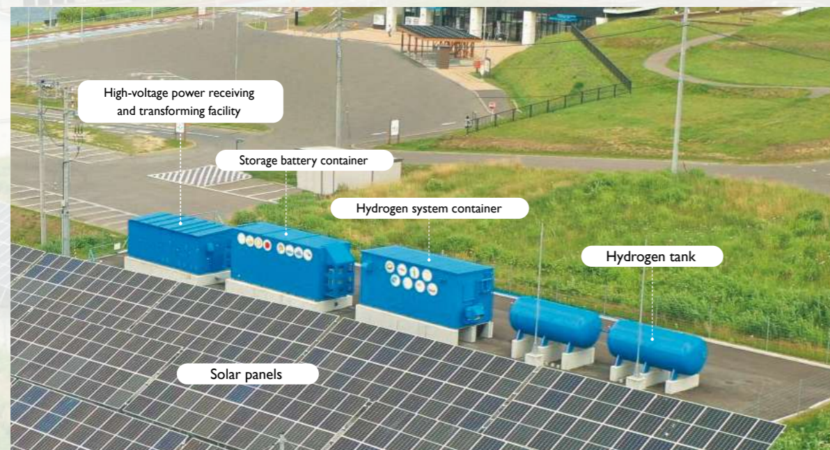
Exterior view of the microgrid system in Atsuta, Ishikari City (Photograph courtesy of Ishikari City)
