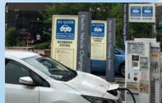
EV charging stations
