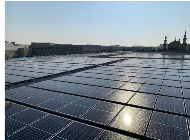
Additional solar panels installed within our premises
