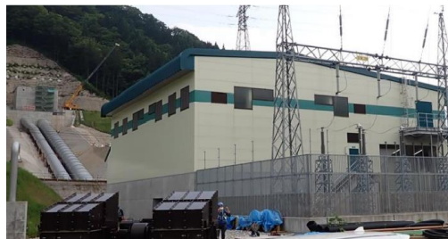
【Tamagawa No.2 Hydroelectric】 Output 14,600kW (Operation Date:Nov.7 2022) Construction using funds procured through green finance
