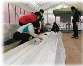
Covering the bed with waterproof, water supplying, and root barrier sheets, and spreading pumice on top of the sheets
