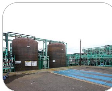
Seki Business Office (water treatment)
