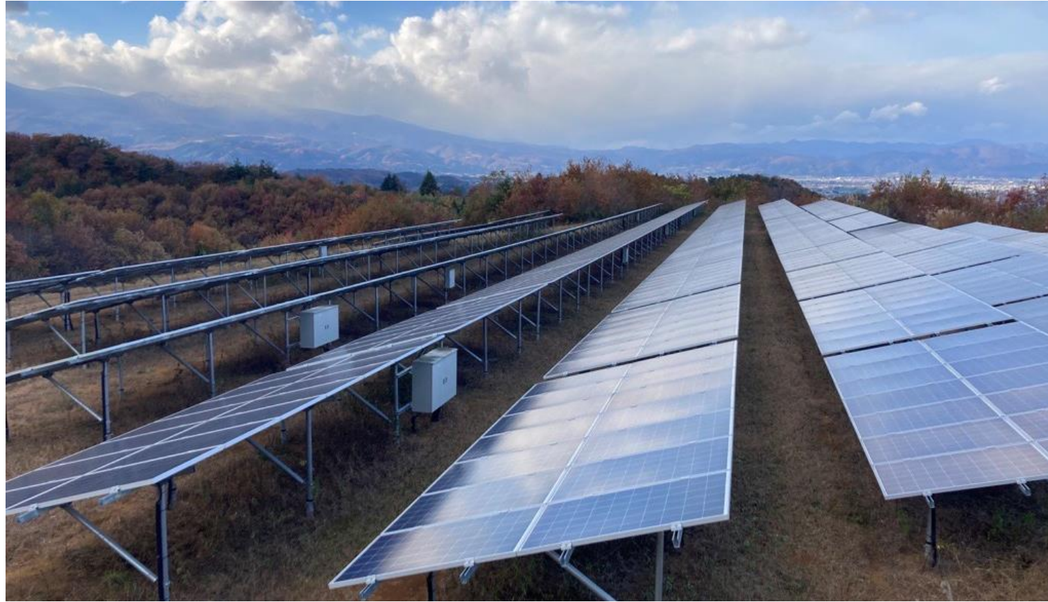
(TESS Fukushima Tazawa Solar Plant)
