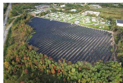
Solar power plant developed by Summit Ridge Energy, LLC (Maine, US)
