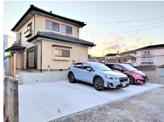
Removed the gate and front yard to create four parallel parking spaces that can comfortably accommodate visitors.
