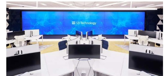
Security Monitoring Centre
