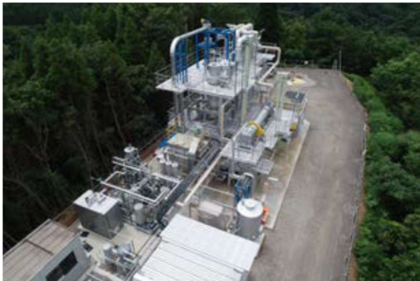
A completed hydrogen production demonstration plant in the town of Kokonoe, Kusu District, Oita Prefecture
