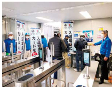
Activities at the gate at Toranomon-Azabudai District Redevelopment Project for A District Project
