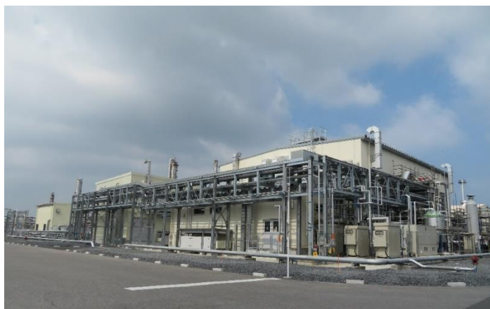
Appearance of Plant 1 scheduled for increasing the capacity
