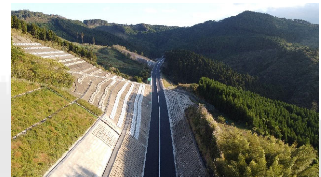
Pavement work near Akagi area (Kiyotake to Kitago) on Higashi Kyushu Expressway
