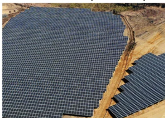
Hanabatake Solar Power Plant (Gunma Prefecture)
