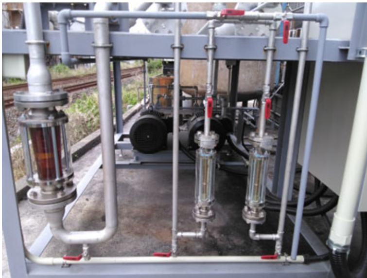
Bio-Diesel Fuel Membrane Separation Type Refinement Test Plant
