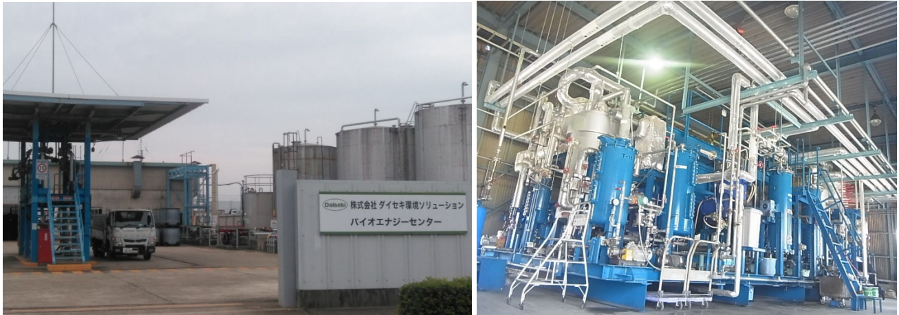
Daiseki Eco. Solution Bio Energy Center in which membrane separation facilities are to be installed (Tokai, Aichi Prefecture)
