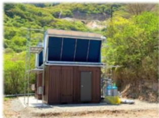
Hakone Yunohana Prince Hotel binary power generation facility
