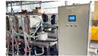
Control of biomass power generation
