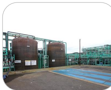
Seki Business Office (water treatment)
