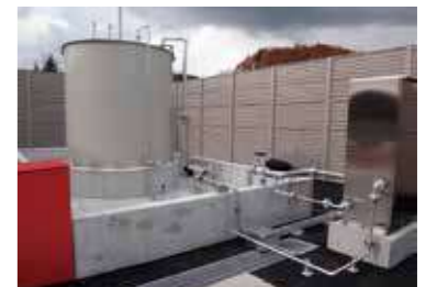
When all of Hokkaido experienced roughly two days of power outage due to the earthquake that occurred on September 6, 2018, our production plants and logistics facilities in Hokkaido continued to operate normally by using emergency power generation equipment.
