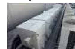
Ice storage air conditioning system
