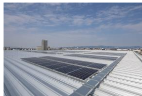
Rooftop solar panels
