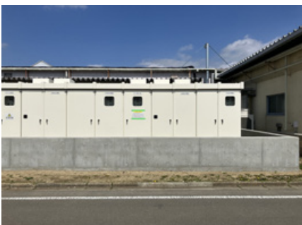
High-voltage power receiving equipment; retaining walls (RI Tohoku)
