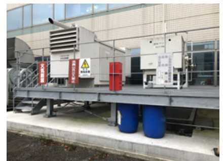
Emergency generator raised off ground (RTC)
