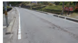
Damaged road pavement
