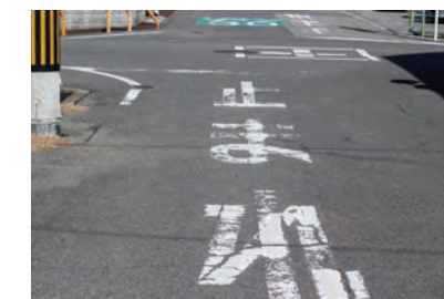
Worn road markings
