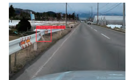
Damage to a guardrail
