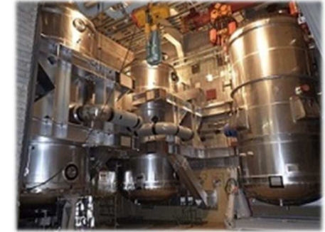
Onagawa Nuclear Power Station
