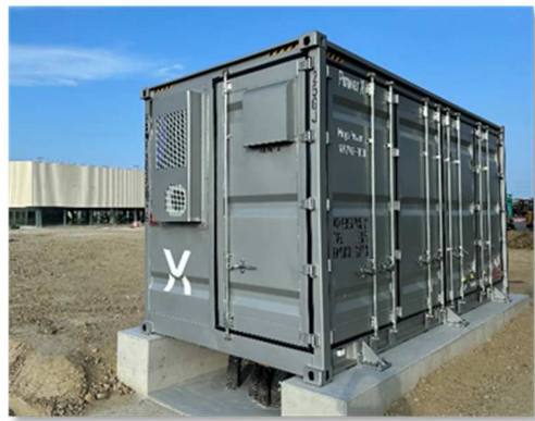
PowerX Inc. Stationary storage battery "Mega Power" (Okayama storage battery factory)
