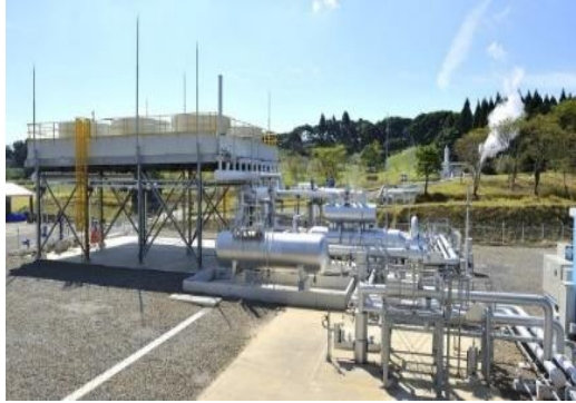
[Geothermal Power Plant in Medipolis Ibusuki]
