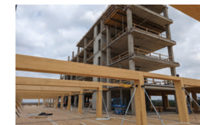
Construction site of a wooden office building in the suburbs of Dallas (taken May 11, 2023)
