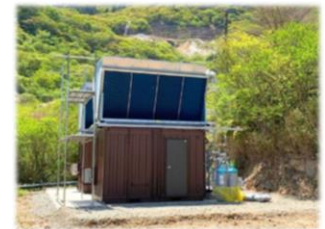
Hakone Yunohana Prince Hotel binary power generation facility
