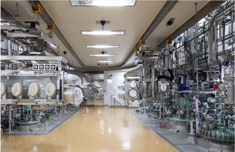
Envisioned processing facilities in FJ2
