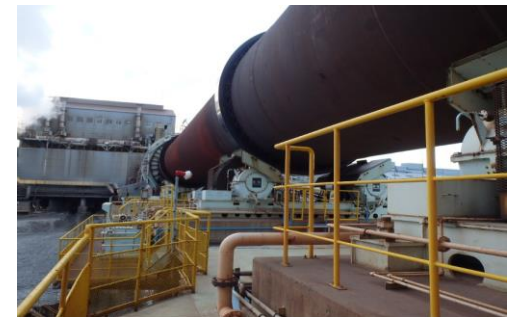
Rotary kiln in operation (at PAMCO)
