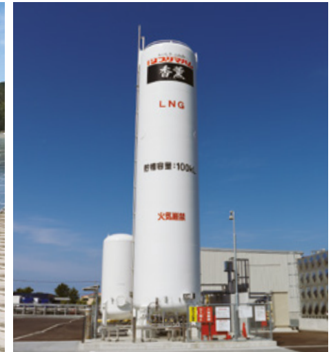
For boiler fuel, the plant uses LNG, which has a low carbon footprint.
