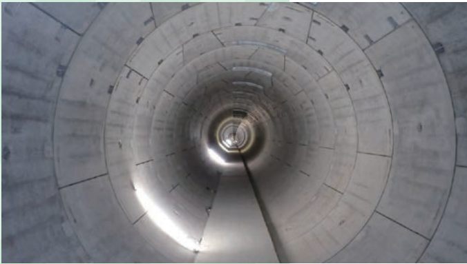
National Route 20 Chofu (2) multi-utility pipeline.
