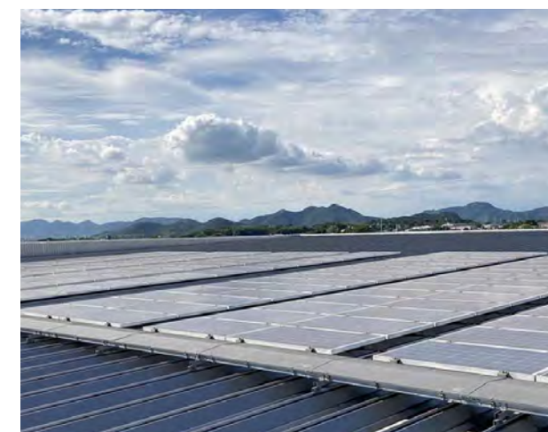
Solar panels (i-Square)
