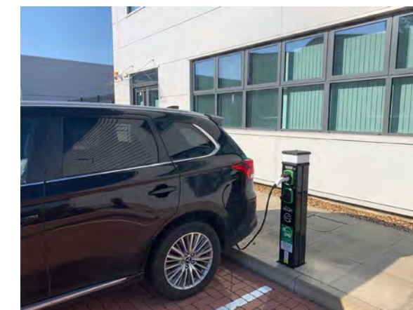
Charging point (Systemex UK)
