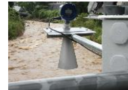
Level gauge that monitors river flooding
