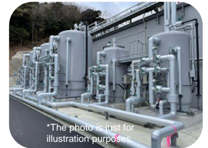
Operation start scheduled in April 2026 New water treatment facility
