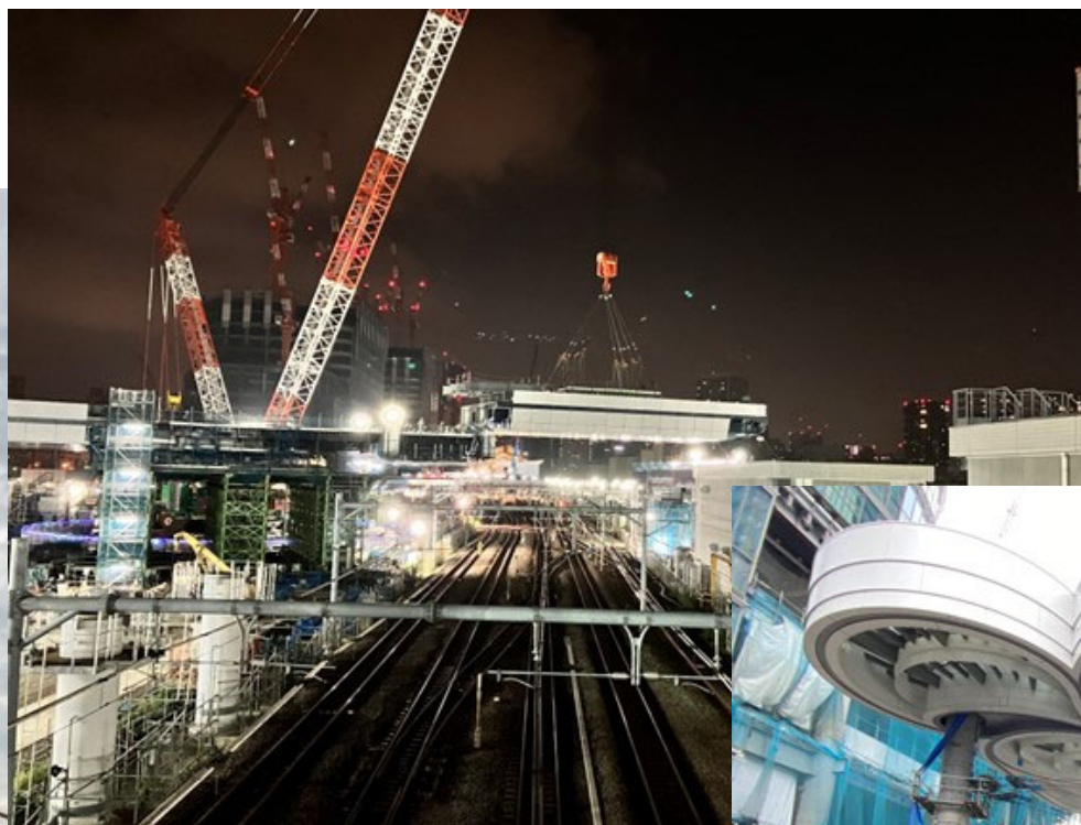
New construction of crossing section of Kanjo 4 Expressway within Shinagawa Station building, etc. Kajima Corporation
