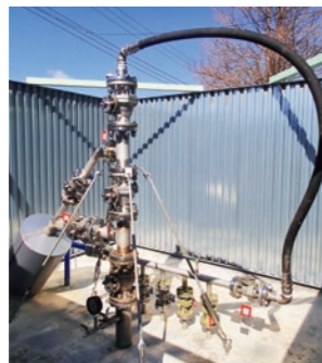
Well for extracting brine water and natural gas
