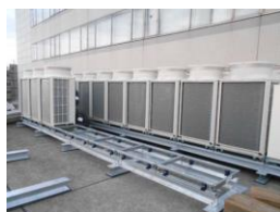
Renewal of air-conditioning system
