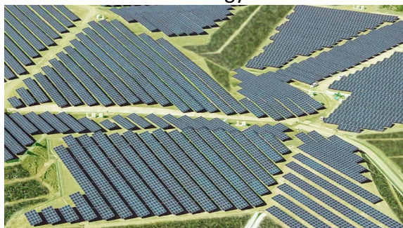
Kakuda City Solar Power Plant/ (DC) 18.3MW
