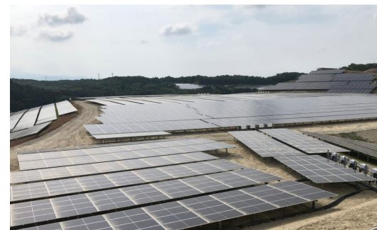
Taiwa Town Solar Power Plant/ (DC) 10.8MW
