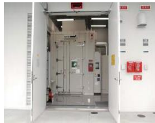
Walk-in Type Temperature & Humidity Chamber for charge-discharge testing
