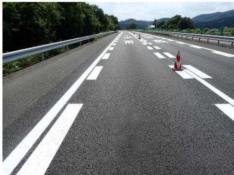
Pavement repair work within the jurisdiction of Utsunomiya Operation Office of the Tohoku Expressway
