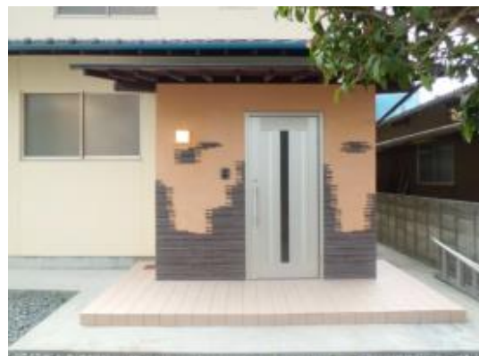
House where porch tiles were replaced, a new exit door was installed and the exterior wall was clad with accent tiles
