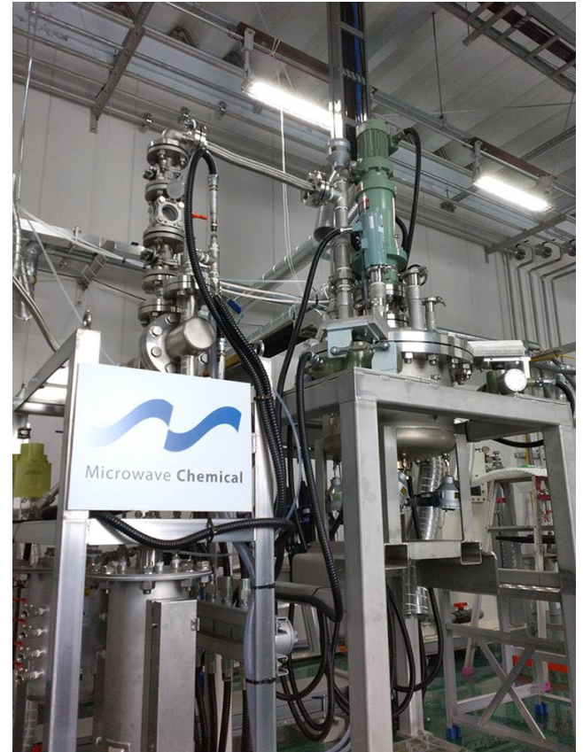
The bench plant used for verification and testing
