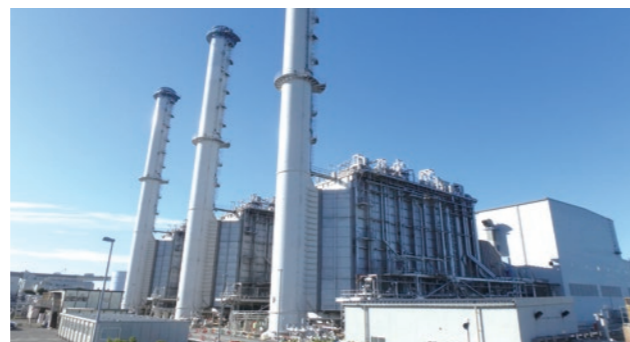
Ohgishima Power Station
